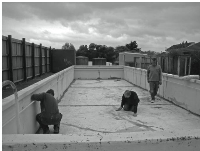
Pool repairs underway by Shirley Intermediate Board of Trustees Chairperson Kevin McDonald, assisted by swim club committee members: Roger Dowling and Paul Somerville.
